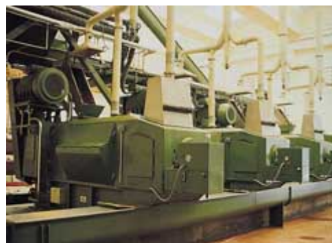
Presses continues (Photo TREMESA SA. )
